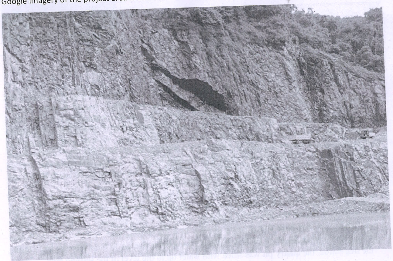
Fig.2 Fracture pattern on quarry wall.
